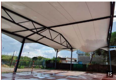
Figure 15. Flat panels and rigid edges lead to ponding.
