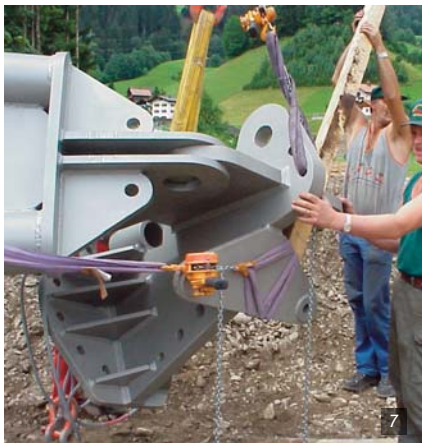
Figure 7: Ice Skating Ring, Montafon. Attachment of holding devices and tensioning equipment (Courtesy of R.Off).
