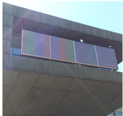
Figure 9: Installation of 4 modules of the prototype on ITMA premises in Pamplona, Spain [1]
