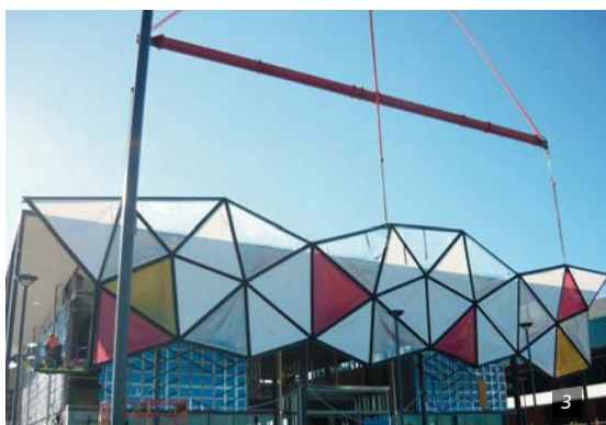
Figure 1. Colourful ETFE façade as a huge lampshade © Kevin Chamberlain Figure 2. ETFE façade as second layer installed 3m in front of the main glass wall © Kevin Chamberlain Figure 3. Installation of the colourful ETFE façade as an artistic solar barrier © Kevin Chamberlain
